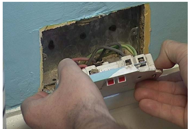
Socket-outlet with broken face plate
