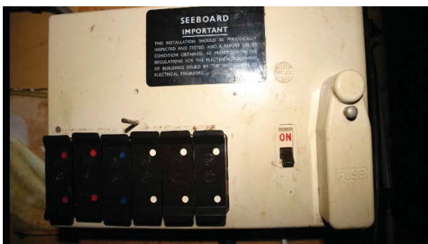
Consumer units having rewirable fuses can continue to provide satisfactory service
