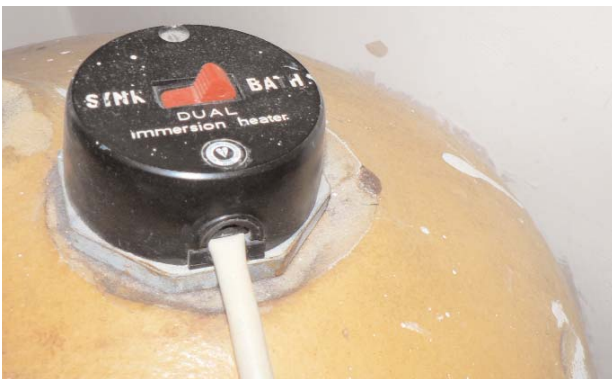
Older immersion heater without thermal cut-out
