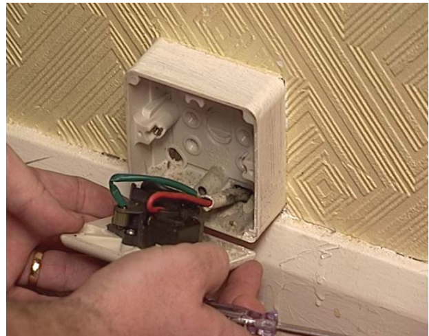
Inspecting a socket-outlet
