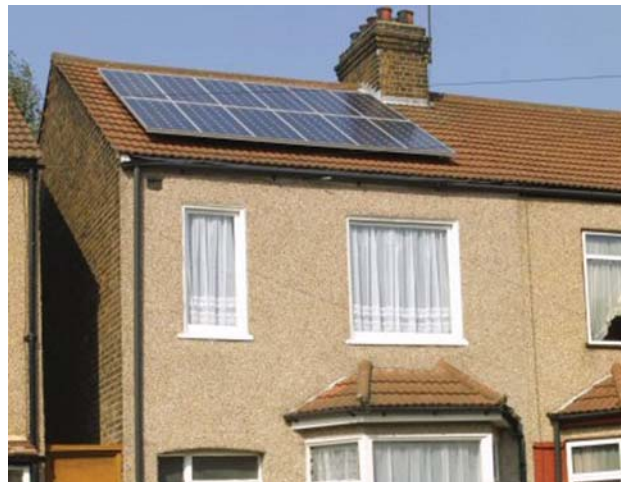
Photovoltaic installation (photo courtesy Energy Saving Trust)
