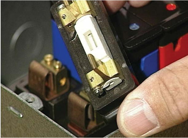
Checking a fuse carrier
