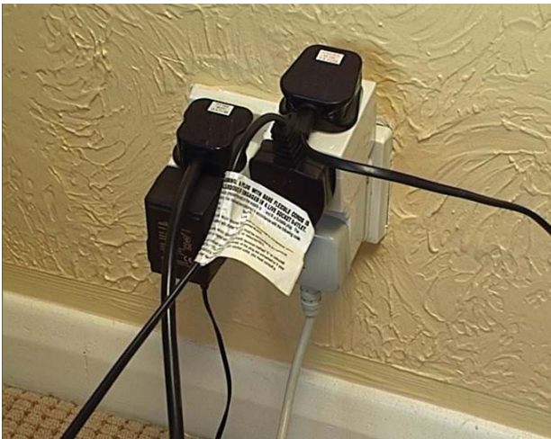
Potentially overloaded socket-outlet
