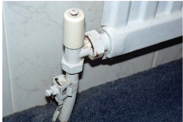
Unmarked bonding conductor
