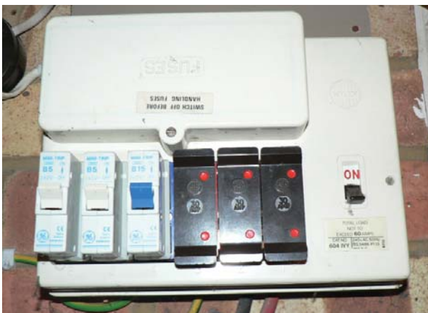
Consumer unit with fuses and circuit-breakers
