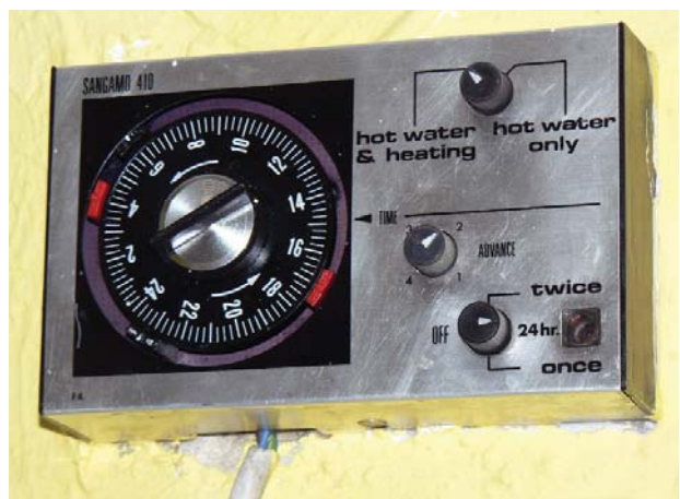
Cable sheath not taken inside enclosure
